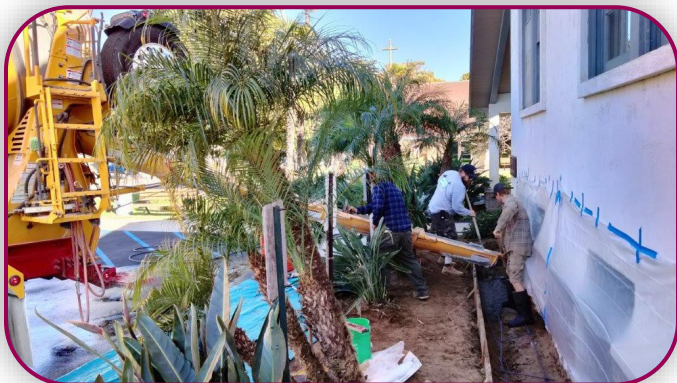
Labor of Love: Pouring the Cement Foundation for the New Screen in Front of the Admin. Building. Photo by Mark B.
